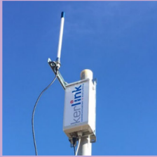
LoRa WAN antenna and gateway
